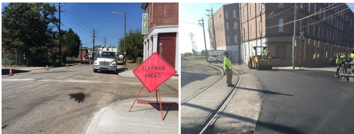
Fig. 5.8. Field view of mill and overlay on Portland Avenue in Louisville, KY
