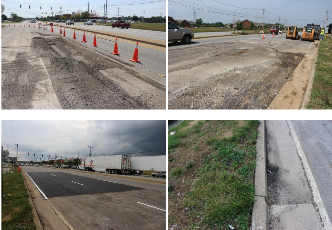
Fig. 5.2. Field view of utility cut restoration on Fern Valley Road in Louisville, KY
