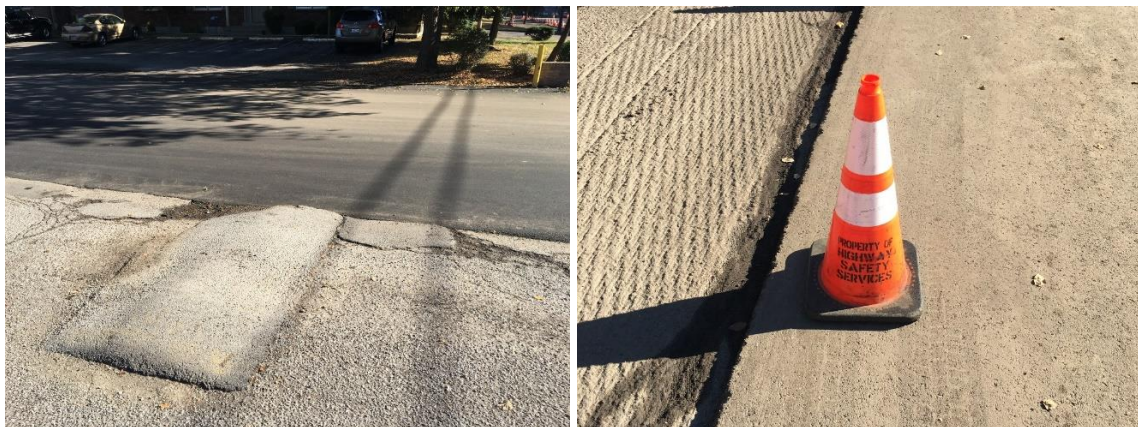
Fig. 5.9. Field view of mill and overlay on Craft Drive and Quest Drive in Louisville, KY
